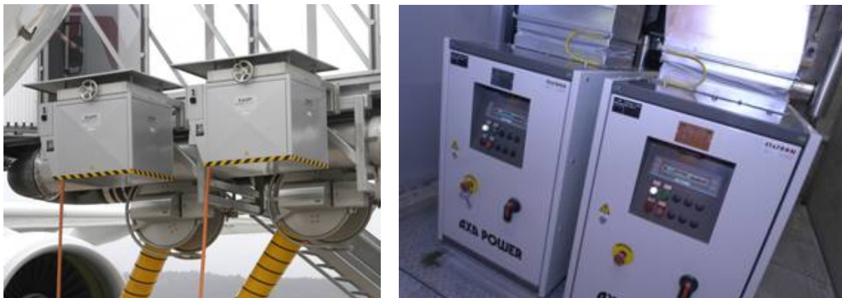
Figure 6 Cable and hose coils (left) and 400Hz transformers (right)
