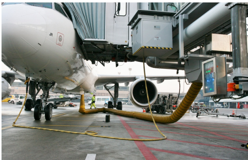
Figure 5 Hose for pre-conditioned air at pier B.
