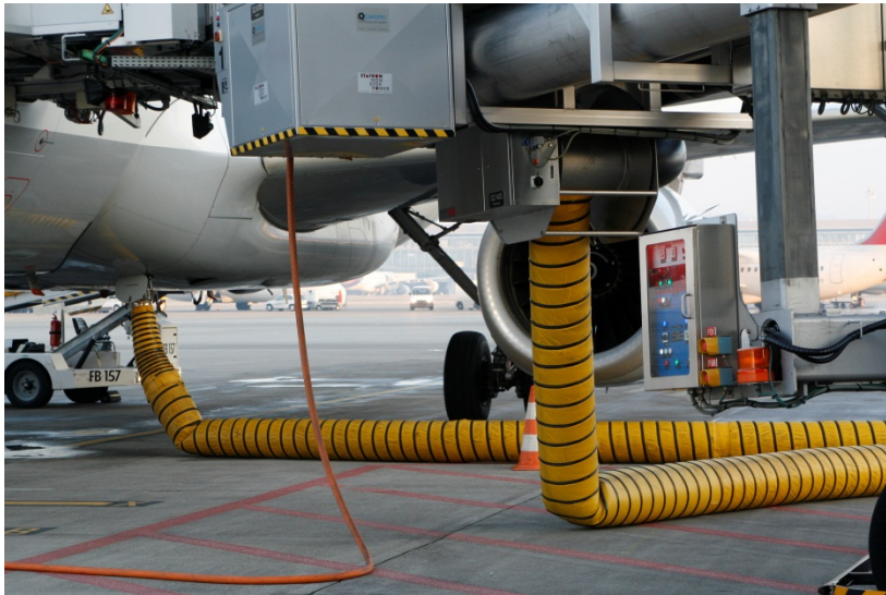
Figure 4 Hose for pre-conditioned air at pier A.
