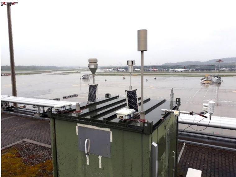
Figure 4 Reference station roof Pier A in top of the Air Quality Station
